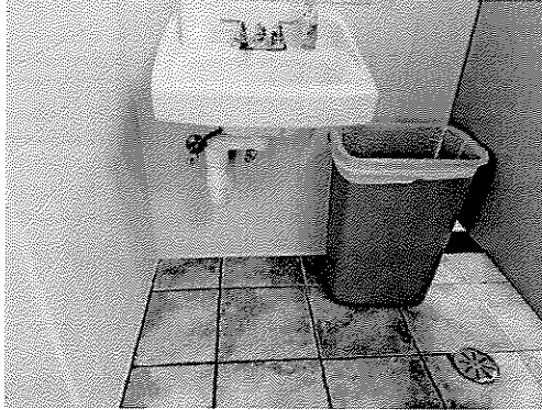
Bathroom sink with pipe cover
