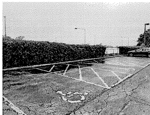
ADA parking without signage
