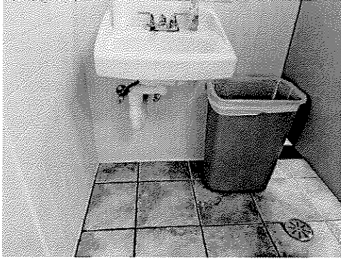
Bathroom sink with pipe cover
