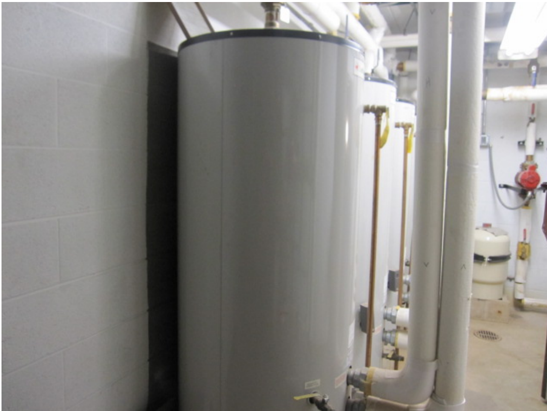
View of the Boiler Room
